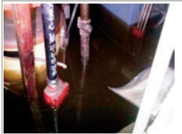
A basement water heater and other equipment are nearly submerged by storm surge.—Photo courtesy of SRNY
