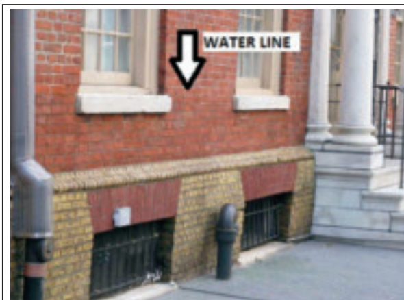
Flood waters outside reached windowsill level. —Photo courtesy SRNY
